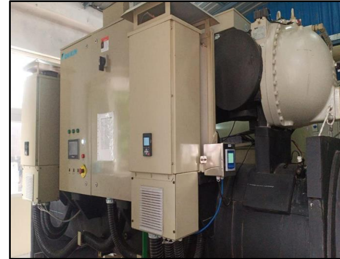
350 TR WATER COOLED SCREW CHILLER
