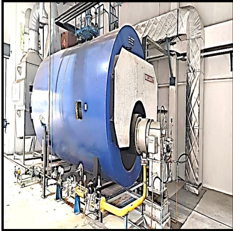
6 TPH PNG/ HSD FIRED BOILER
