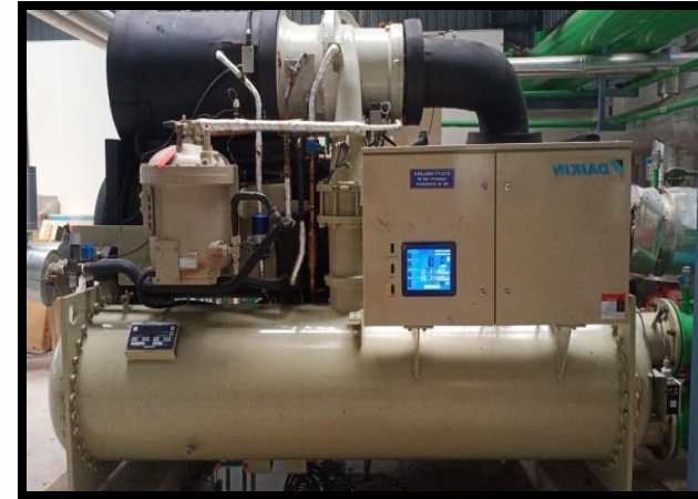
450 TR WATER COOLED SCREW CHILLER
