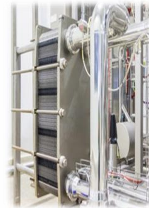
Plate Heat Exchanger installed at boiler feed water line
